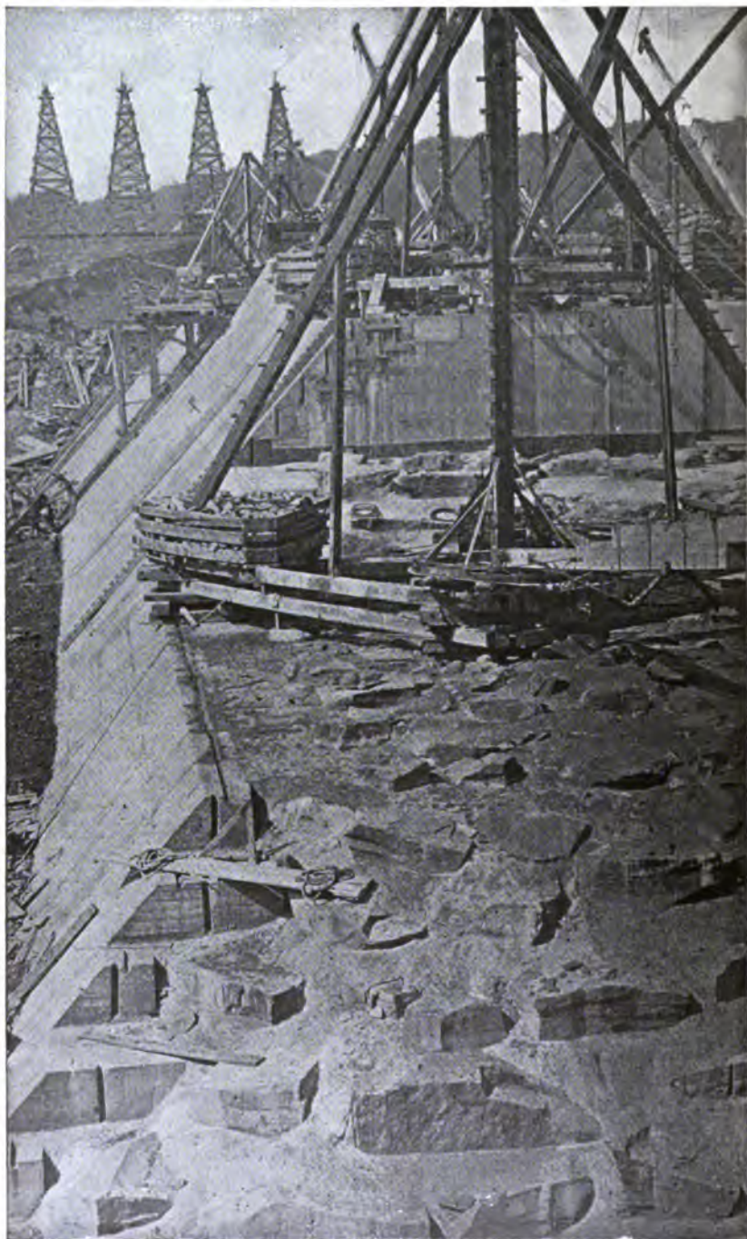
PLATE 40. —View of Partially Completed Olive Bridge Dam, Showing Concrete Facing Blocks, Cyclopean Masonry, Cableways, and Derricks Used in Placing Masonry; also Transverse Expansion Joint Across Dam.
